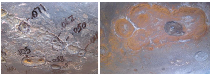
Fig. 6.2 Two examples of MIC-related failure featured as pit-in-pit in a carbon steel pipeline’s external surface that had both coating and under CP and buried in a soil with pH of 5.5. © NACE International 2013
