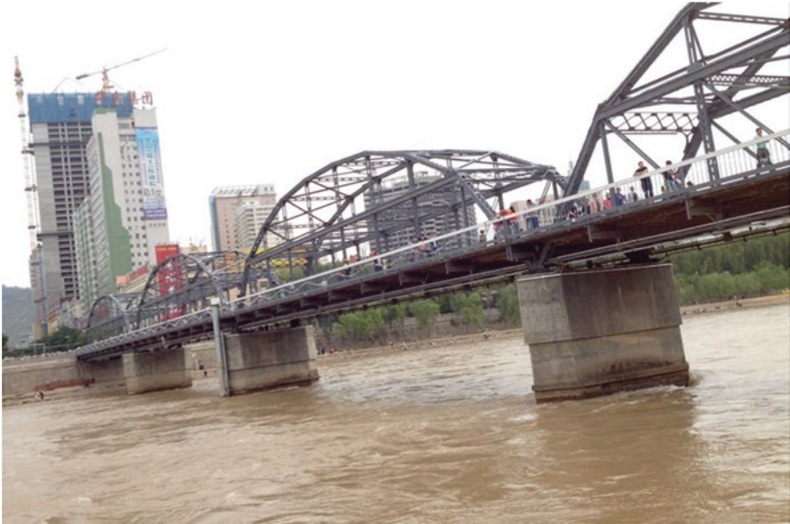
Fig. 4.8 Iron bridge over the Yellow River in Lanzhou City, China (Photo by Zhanhuan Shang)
