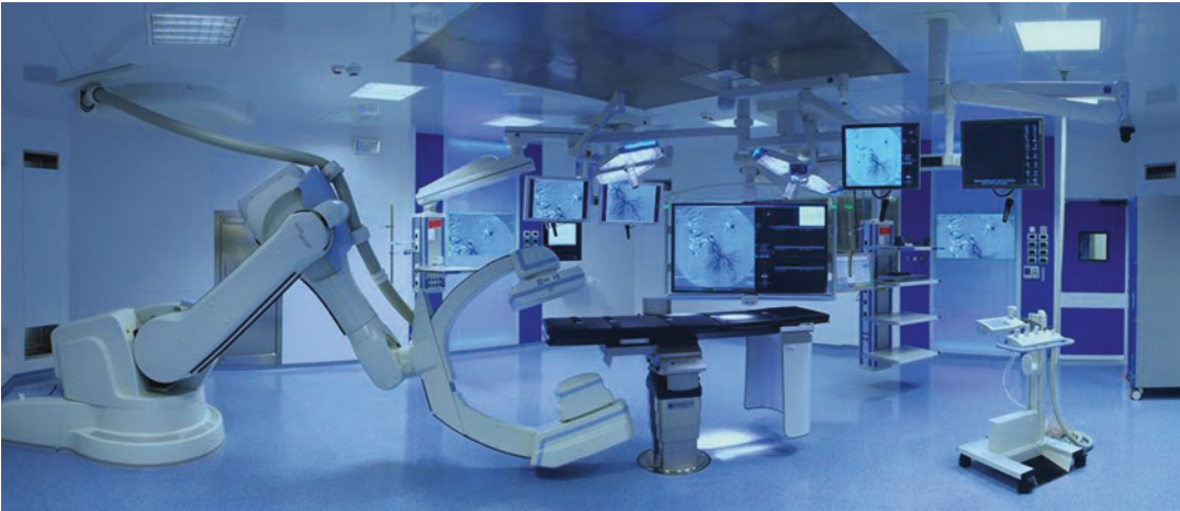
Fig. 12.2 New Hybrid Operating Room, Rome, Italy
