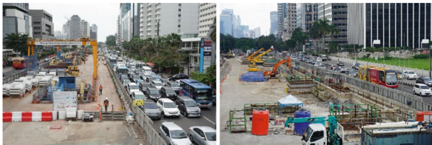
Fig. 6.11 Construction works for the new Mass Rapid Transit system. Photo courtesy of Muhamad Rizki
