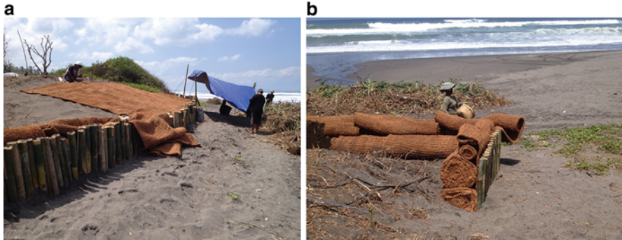
Fig. 20.8 Pictures of the on-site coir geotextile installation: (a). shows the cross-sectional view on the textiles; (b). shows the bamboo wall and the installation of the top coir layer © David 2014
