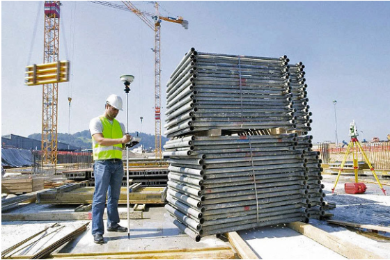
Fig. 35.11 GNSS as typically used by surveyors on construction sites: here is shown a pole-mounted GNSS receiver which is being used to either coordinate a point-of-interest or to mark a point whose coordinate is provided in order to set out formwork for concrete pouring, laying of cables, pipes, or services, etc.; typically operating in real-time mode (courtesy of Leica Geosystems)
