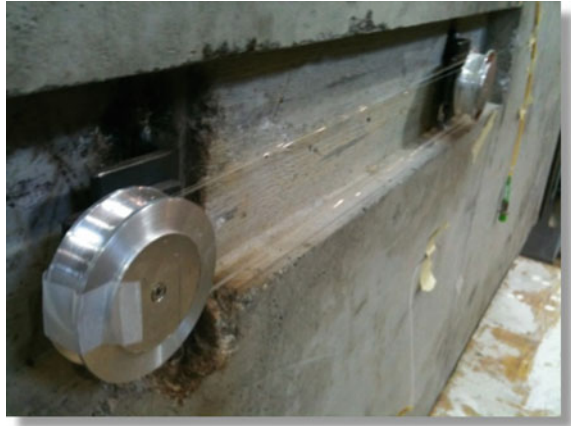
Fig. 7 Brillouin Sensors installed at test tunnel perimeter. MONICO (FP7) EC co-funded research project [7]
