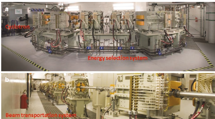
Fig. 2.1 Cyclotron and energy selection system (a) and a section of the beam transportation system (b) for a proton therapy facility (Courtesy of IBA, SA). Vacuum tube with multiple steering or bending magnets guide and focus the narrow proton beam to treatment rooms
