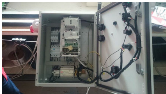
Fig. 3 View of control box
