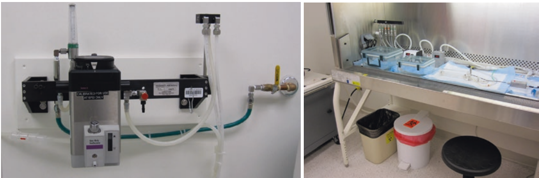
Fig. 3.8 Wall mounted gas anesthesia systems keep the counterspace clear, are easy to use and provide a constant depth of anesthesia ( left image ). This single cost effective system provides anesthetic gas to multiple induction boxes and nose cones in a biosafety cabinet ( right image ),
