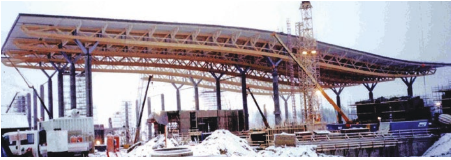
Fig. 5 Glulam trusses of extremely large span used in roof structure of the Oslo-Gardermoen airport. Trusses are mounted on tall post-tensioned concrete columns ( Photo R. Tarczewski )
