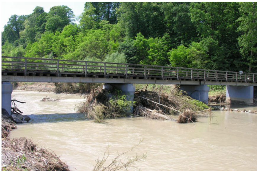
Fig. 4 Partial clogging of the bridge at Jankowa on the Biała River with large woody debris trapped on the bridge pillar during the flood of June 2010. The bridge clogging directed the flood flow onto the adjacent valley floor, causing flood damage to the nearby houses and infrastructure
