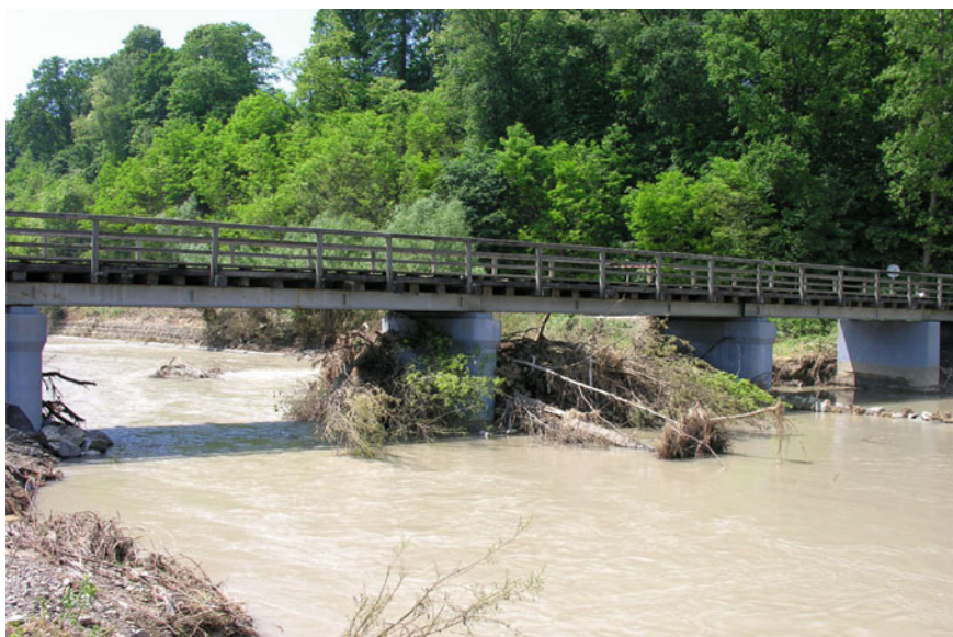
Fig. 4 Partial clogging of the bridge at Jankowa on the Biała River with large woody debris trapped on the bridge pillar during the flood of June 2010. The bridge clogging directed the flood flow onto the adjacent valley floor, causing flood damage to the nearby houses and infrastructure
