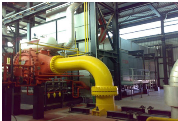
Fig. 2 Examined gas turbine GE 3002
