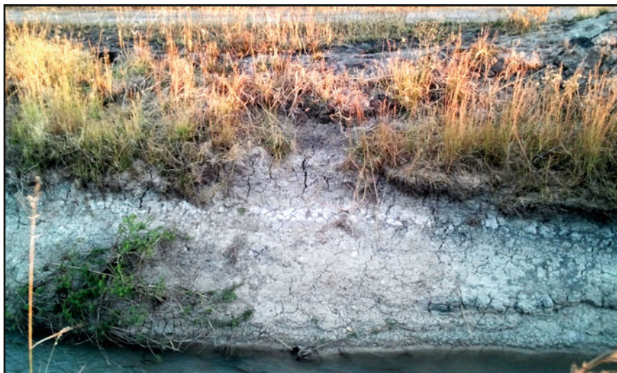
Fig. 6.8 Water drainage canal with strong salty symptom in Madibira Irrigation Scheme, Mbeya, 2014
