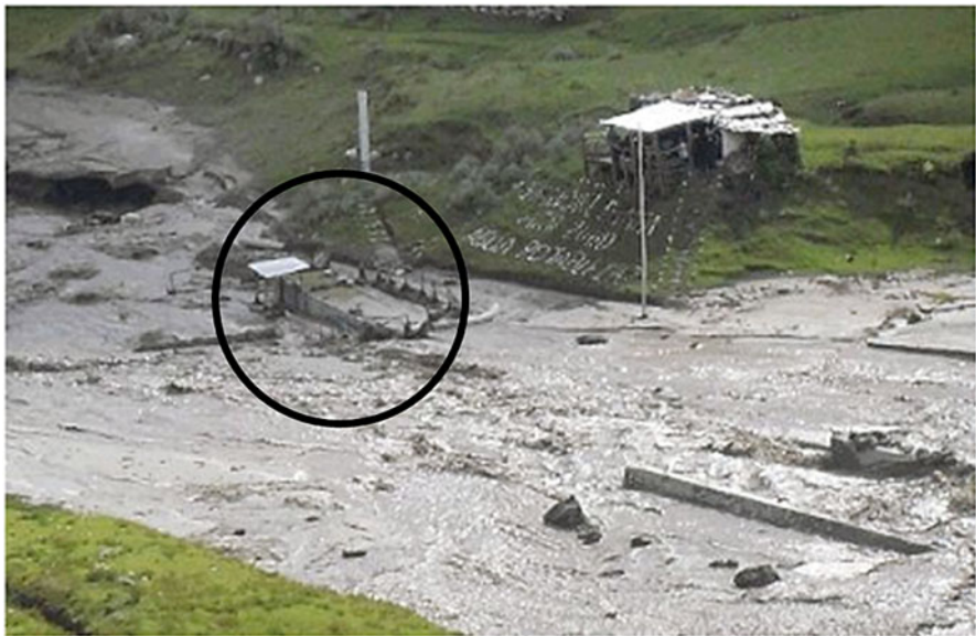
Fig. 4 Hyperconcentrated flow on the Shonquillpampa during the April 2010 GLOF. In the circle the plant of drinking water for the city of Carhuaz that was partially damaged
