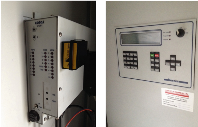
(a) Battery pack connected (b) Front picture ground controller
