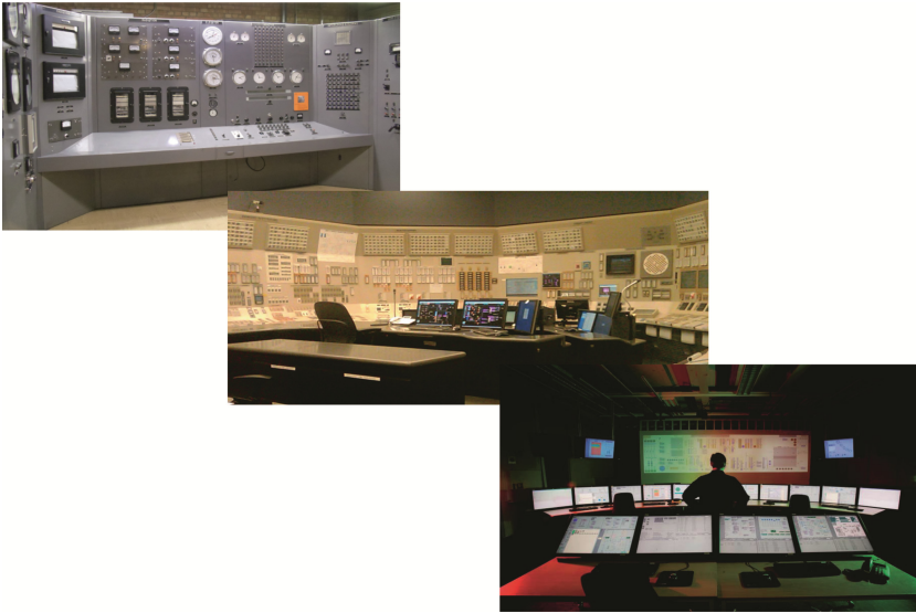
Fig. 1. Three generations of nuclear power plant control rooms (top to bottom: EBR-1, the first nuclear power plant with an all analog control room; recently decommissioned San Onofre Nuclear Generating Station, with a hybrid analog-digital control room; HAMMLab at Halden Reactor Project, a fully digital advanced control room concept).
