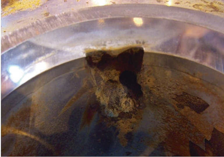
Fig. 11.12 Damage to seat of the second bypass valve
