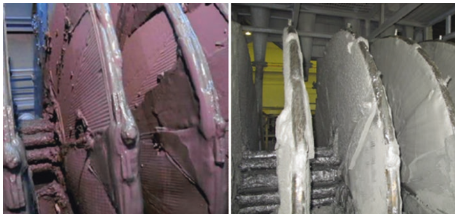
Fig. 5.11 Disc filters for dewatering full plant ( left ) and cycloned ( right ) tailings slurries
