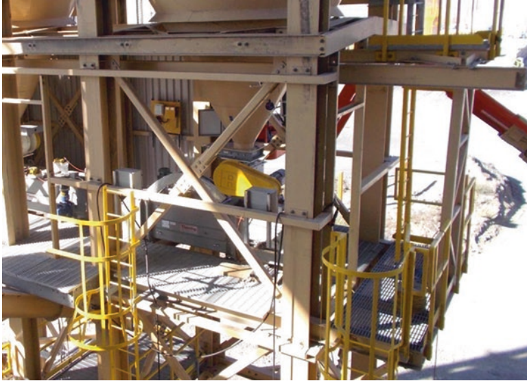
Fig. 12.3 Illustration of the binder silo bottom cone where the rotary valve discharges to the binder weigh conveyor; picture taken during construction
