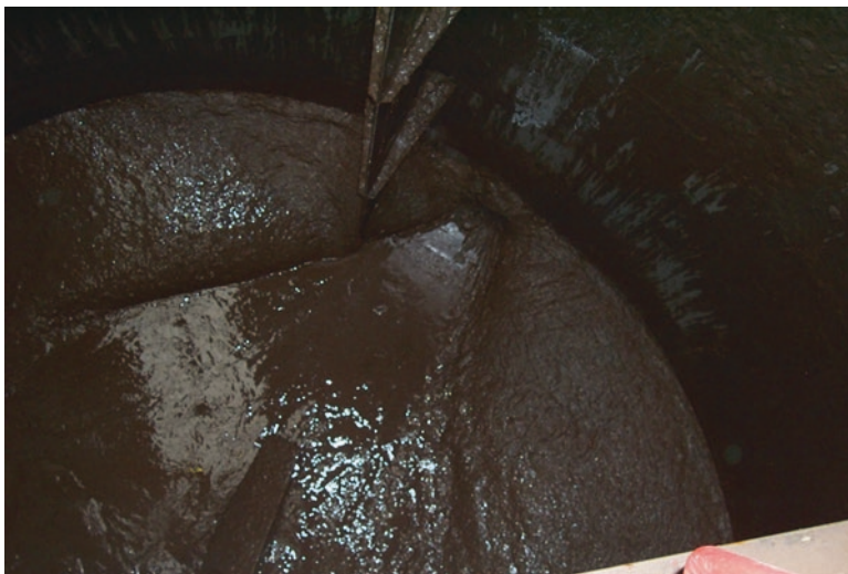
Fig. 11.15 Build-up in backfill tank following draining for inspection
