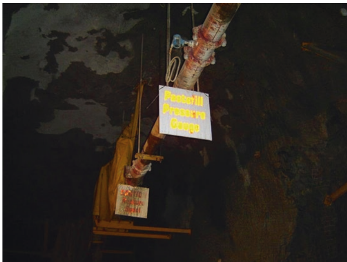
Fig. 7.3 A pressure transmitter installed on an underground distribution system to monitor pipeline pressure at specific locations. A rupture spool can also be seen in the background
