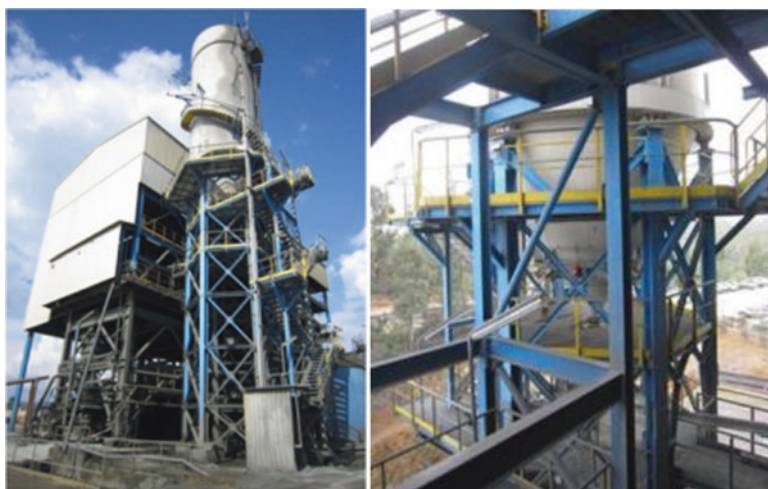
Fig. 5.13 A 350-ton cement storage silo considered for paste backfill plants
