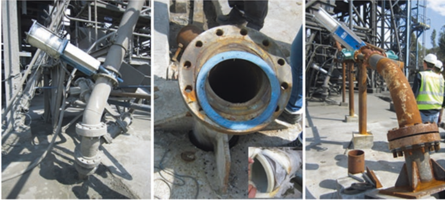
Fig. 5.15 Photos of the borehole system for paste backfill transport to underground mines
