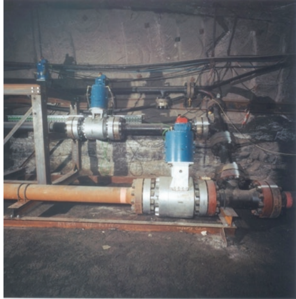
Fig. 11.9 Underground valve station
