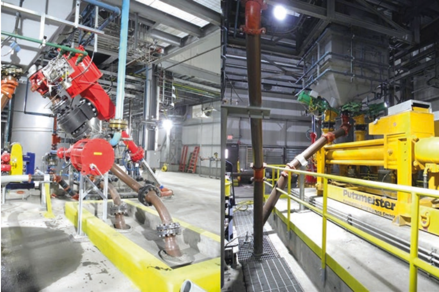
Fig. 12.5 Illustration on the right depicts the paste hopper and its connection to the piston pump. Illustration on the left shows the gravity (foreground) and pumped inclined boreholes. Note that the paste hoppers are outfitted with freshwater line (blue piping) for clean-up
