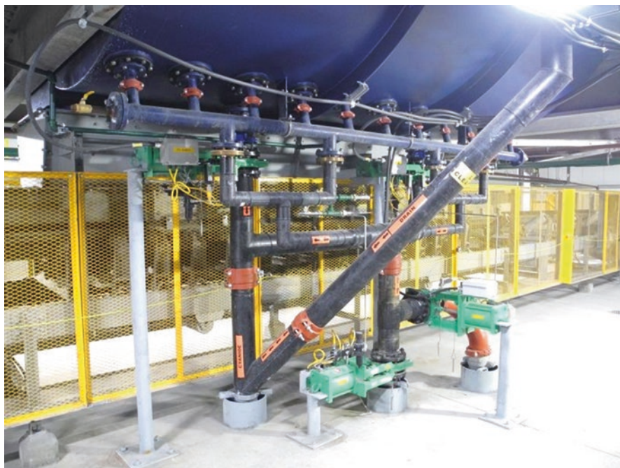
Fig. 12.2 Thickened slurry feed to eductor distribution across the length of the disc filter vat. Overflow and drain lines from the disc filter also shown in larger diameter HDPE piping
