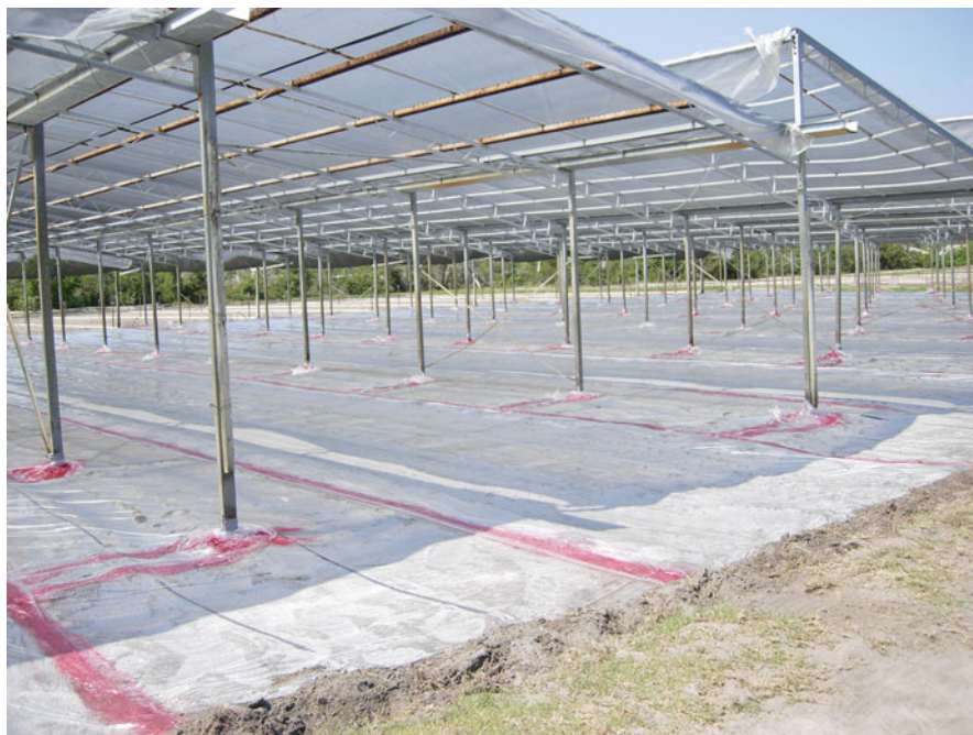
Fig. 7 Soil disinfestation is hampered by permanent infrastructure such as posts for shade cloth and glass (E. Roskopf. USDA.)
