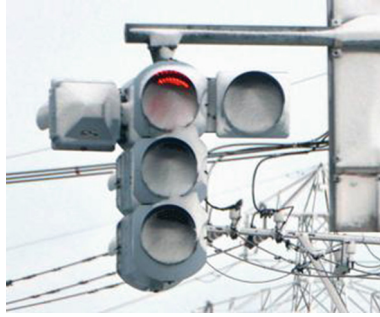
Fig. 5. Heavy snow conditions cover the LED based traffic lamps.
