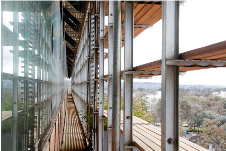
Fig. 1.13 View along integrated access way showing open state of automated upper windows . Image credit Carl Drury
