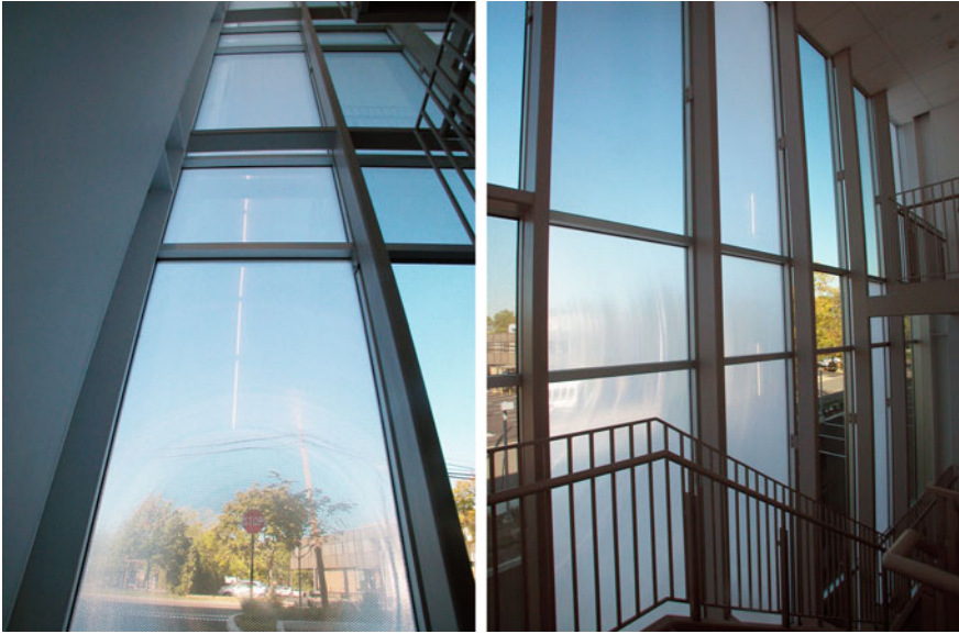
Fig. 3.15 Example views available looking through ClearShade™ installed in exterior curtain wall glazing at INV Management, NJ. Gluckman Mayner architects. Image Credit Panelite
