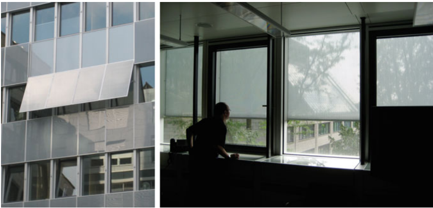
Fig. 2.47 Automated exterior solar control screens applied as a facade retrofit ( revitalisierung ) to the Haupthaus KfW building in Frankfurt ( left ) and interior view with screens deployed ( right )
