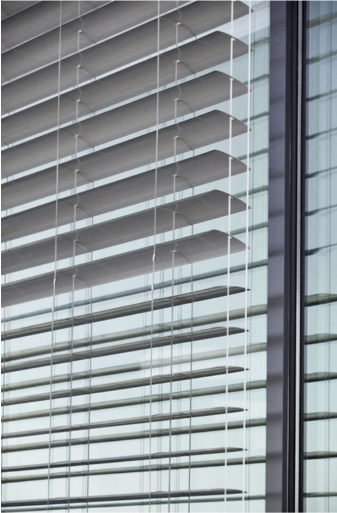
Fig. 5.6 Office/classroom facade ( exterior view ) showing zoned sections of automated venetian blinds. Image credit Behnisch Architekten
