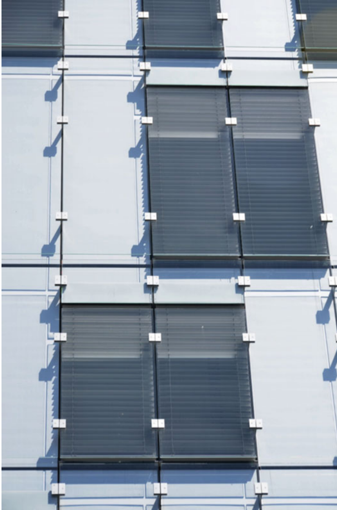
Fig. 5.5 Office/classroom facade showing frameless glass screen wall designed to shield exterior automated venetian blinds. Image credit Behnisch Architekten
