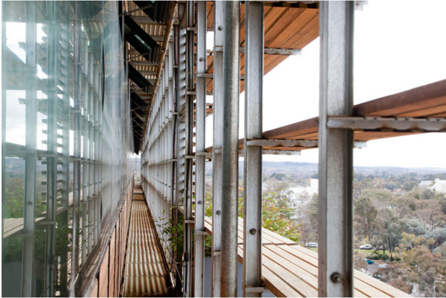
Fig. 5.17 View perpendicular to facade glazing showing external facade shading screen and operable transom windows used for automated natural ventilation. Image credit Carl Drury Photography
