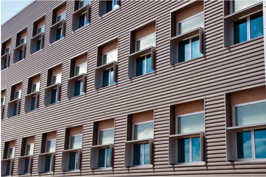
Fig. 5.20 The windows on the south facade are divided into an upper “daylight zone” and lower “view zone.” Exterior shading is designed to provide solar and glare control to the view zone to avoid the need for interior shading devices. This image has been reprinted with permission from National Renewable Energy Laboratory
