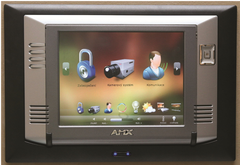
Fig. 3. Intelligent building control panel ca. 2009 [7]
