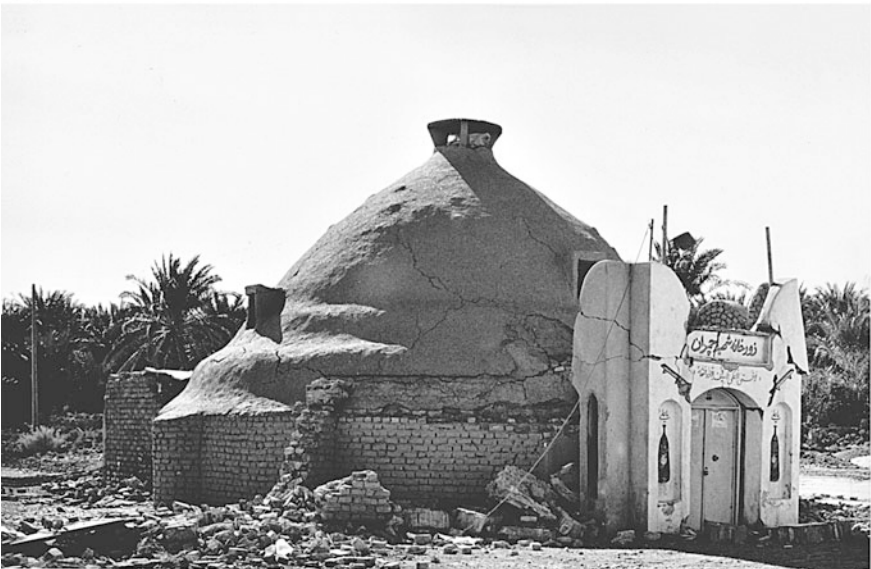
Fig. 6.31 Bam. After the earthquake: a A completely symmetrical mud brick dome belonging to a public bath which has remained safe. b Dome of a gymnasium. A place for traditional athletic exercises, supporting surrounding forms prevented the structure from collapsing
