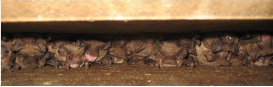
Fig. 9.1 Tightly packed Mexican free-tailed bats roosting in a concrete expansion joint within the Texas A&M football stadium (Kyle field), College Station, Texas, USA
