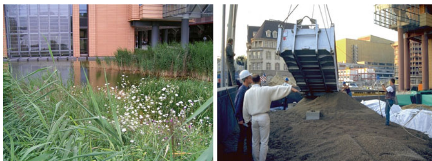
Fig. 19.9 Constructed wetland for rainwater treatment of roof runoff at Potsdamer Platz, Berlin ( left ) and its construction in 1998 ( right ) (Photo author)
