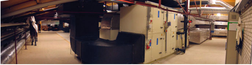
Fig. 9.14 Air handling unit in a mechanical room
