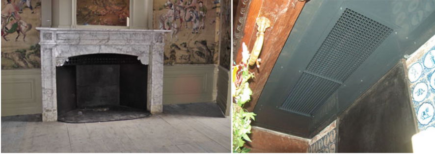
Fig. 9.17 The air inlet hidden in an existing fire place with nozzles to provide a good mixing
