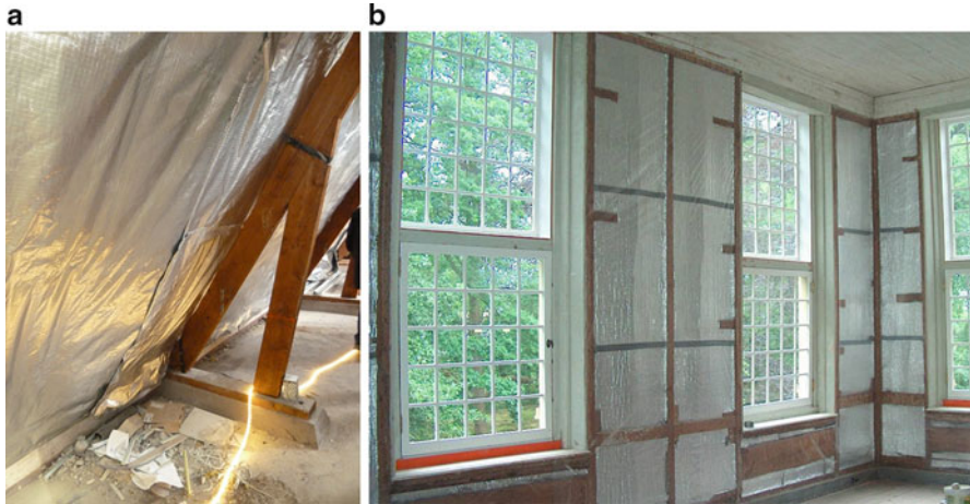
Fig. 7.34 The application of vapor barriers is an import but sometimes difficult job: (a) a vapor barrier with very small overlap and weakly glued seams, this can become problematic in future and needs adjustment (Photo: Van der Wal, Cultural Heritage Agency of the Netherlands), (b) a properly executed vapor barrier with a sufficient overlap and properly glued seams as part of a wall closing protocol
