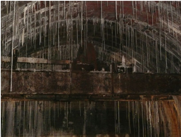
Fig. 5.14 Stalactites made of salts due to water entry through cracks in the bunker complex at the Obersalzberg, Germany
