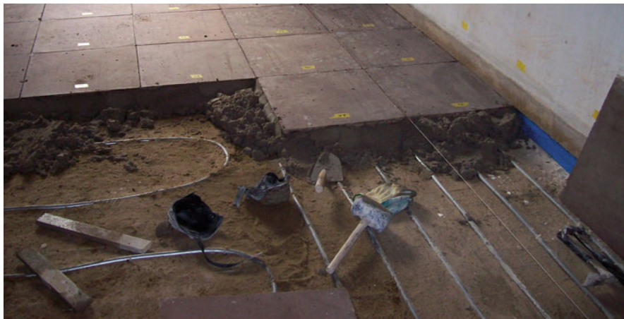
Fig. 10.4 Installing floor heating in the central hall of Amerongen Castle (Photo: Jos Snoek)
