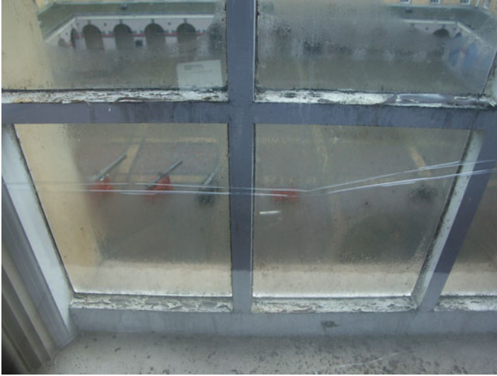
Fig. 9.5 Condensation with subsequent damage of the wooden window frame (Photo: Schonewille, Central Government Real Estate Agency)
