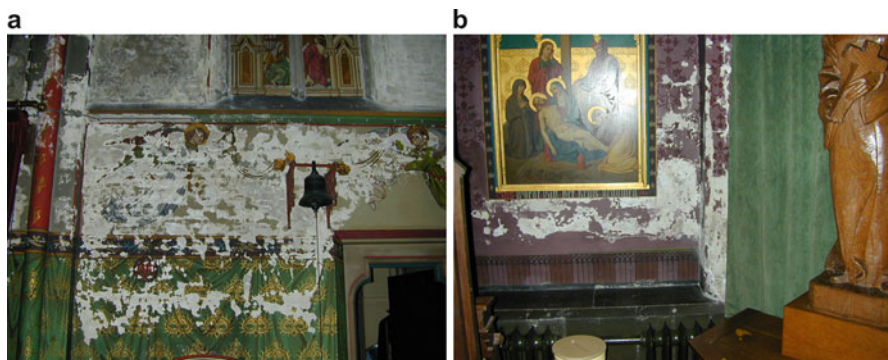
Fig. 5.3 Salt efflorescence near the surface of a catholic church in the Netherlands severely damaging the wall painting (a) and a common cause the heating system (b) near the surface causing high temperatures and low relative humidity
