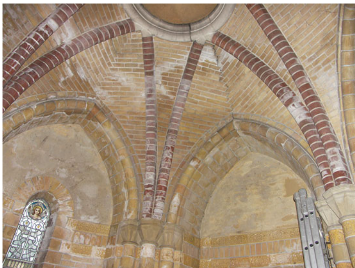
Fig. 5.5 Wet spots on wall due to the absorption of water vapor by local high salt loads in the masonry (Photo: Van Hunen, Cultural Heritage Agency of the Netherlands)
