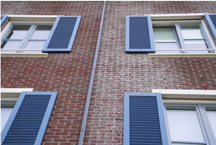
Fig. 5.4 After the construction is complete efflorescence can become visible (Photo: Kemper, FHB Gevelreinigung)
