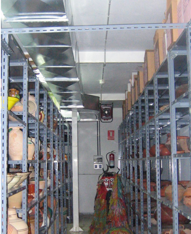
Fig. 9.12 The museum storage in Valle Guerra, Tenerife showing a convective heater on the wall at the far end
