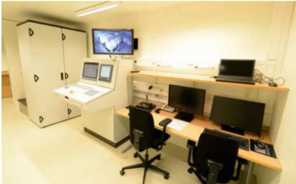
Figure 11 The control room
