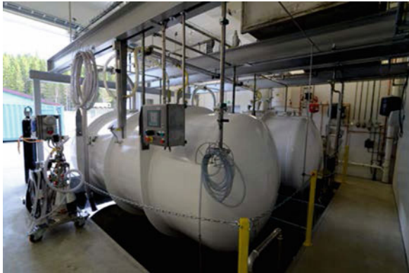
Figure 12 Both tanks in place just above the water basin below floor level
