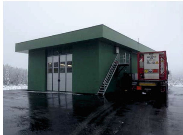
Figure 13 Filling of the tanks from standard truck
