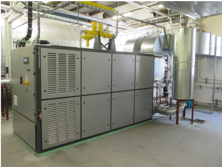
Fig. 4 Cogeneration unit 199 kW e /263 kW
