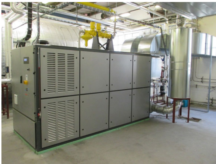
Fig. 4 Cogeneration unit 199 kW e /263 kW
