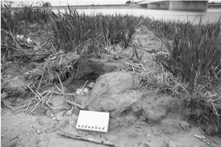
Fig. 4.22 Erosional feature in the lower section of the Natori River (Loc. 1)
