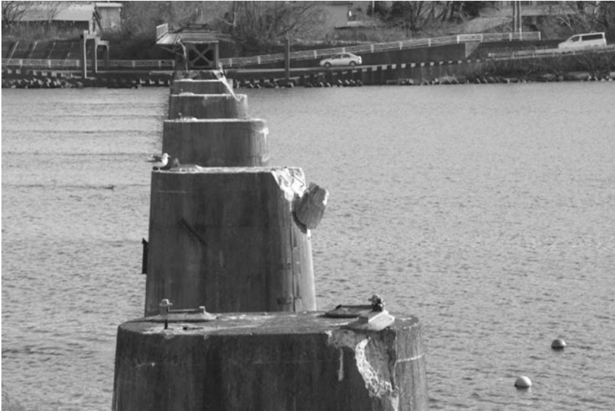
Fig. 4.6 The washed-out railway bridge crossing the Hei River in the Miyako City
