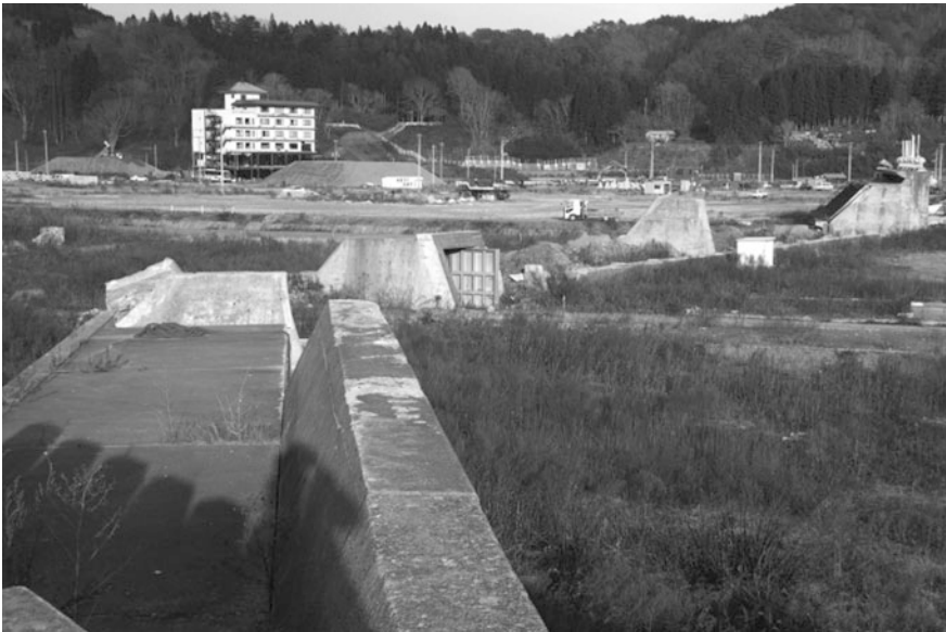
Fig. 4.3 The destroyed mega seawalls of Taro. The upper right seawall was totally washed out. The lower left seawall was quite strong, so that this survived the tsunami overflow
