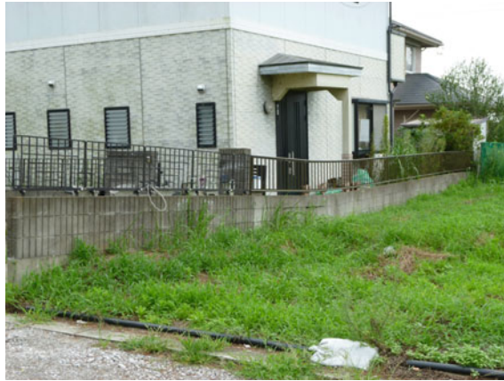
Photo 6.2 Differential settlement landscape at Hinode reclamation area in the former lagoon (taken at July 2011)
