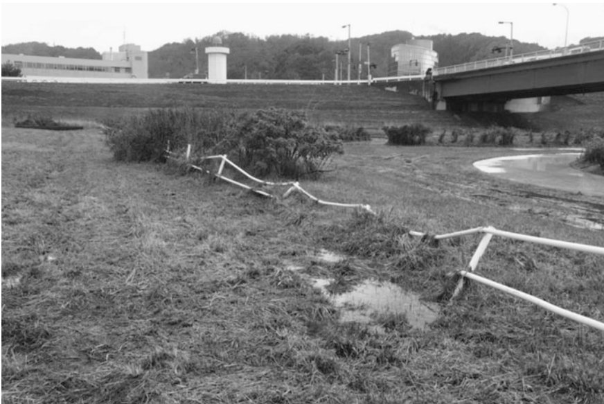
Fig. 4.7 Bended steel fence in the river side floodplain
