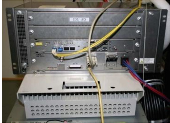
Fig. 12 WiMAX equipment deployed for ORBIT outdoor testbed
