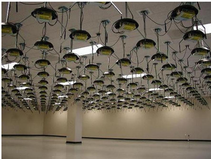
Fig. 2 The ORBIT radio grid deployed at Rutgers Tech Center Facility
