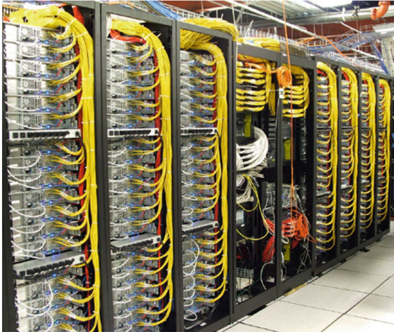
Fig. 2 Wiring in one of the Utah Emulab clusters
