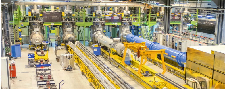
Fig. 1. SM18 Cryogenic Test Facility (©CERN, 2013. CERN-GE-1304099-24)
