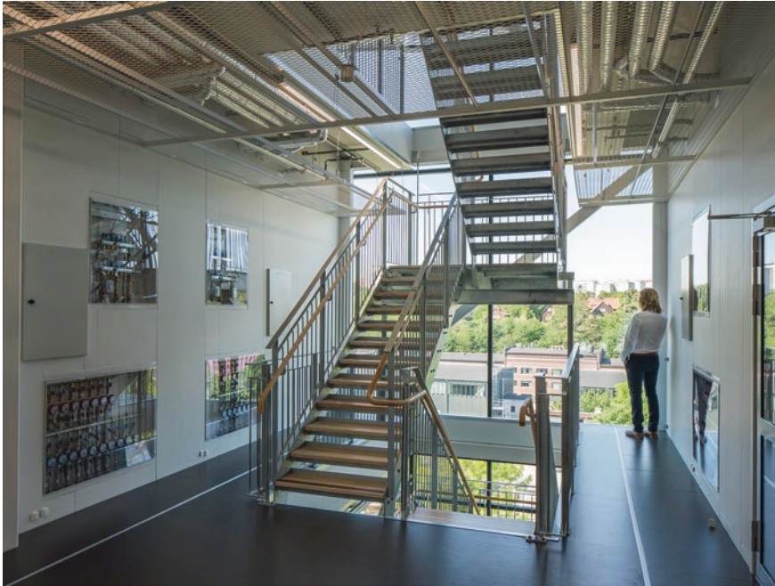
Fig. 10.12 Stairway space of the HSB Living Lab, displaying the unique and transparent, easy accessible, systems
