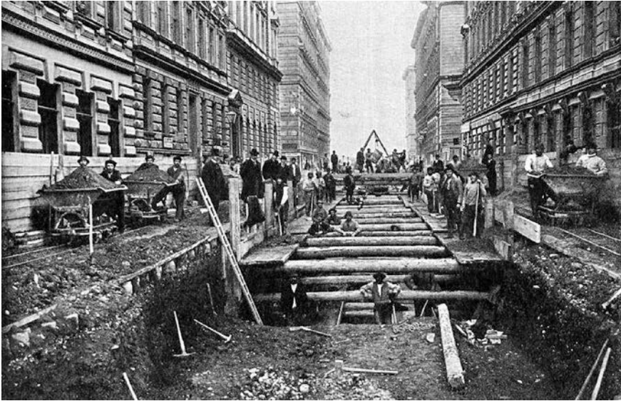
Fig. 24.3 Constructing the main intercepting sewer: construction site on Marxergasse. (Source: Kohl 1905, p. 205)
