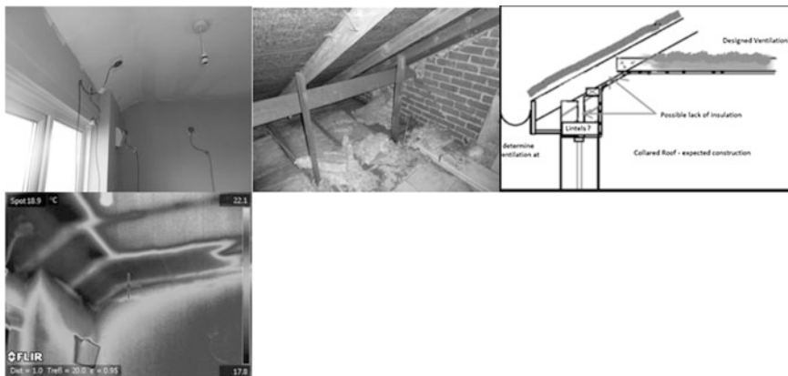
Fig. 11.4 Sloping bedroom soffits. Showing from left to right the bedroom wall, soffit and ceiling; the roof void above showing apparently reasonably laid insulation; section sketch showing thermal bridge position; thermal image of the bedroom wall, soffit and ceiling where the darker sections indicate the thermal bridging
