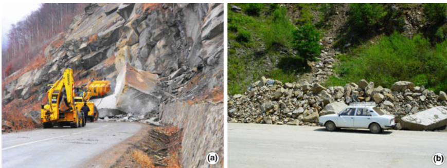
Fig. 11.7 Rockfalls in the Buzău Carpathians, along National Road nr. 10 (Photos M. Micu)
