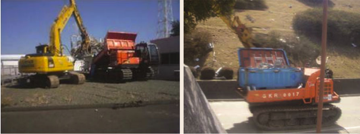
Fig. 60.11a,b Unmanned construction machines used at Fukushima-Daiichi (courtesy of Unmanned Construction Machines Association)
