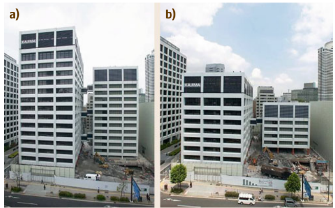
Fig. 57.31a,b Systemic and automated floor-by-floor building deconstruction, Kajima, DARUMA System, Japan (a) early deconstruction phase; (b) later deconstruction phase
