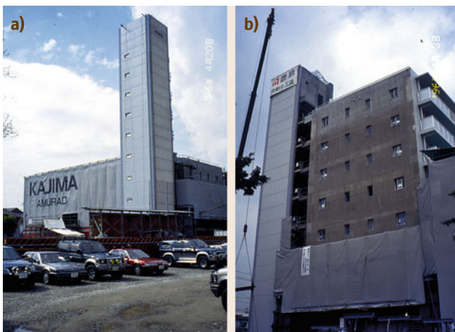
Fig. 57.30a,b The AMURAD Construction Strategy: floor-wise up-pushing of the whole building. Kajima, Japan (a) early construction phase; (b) later construction phase
