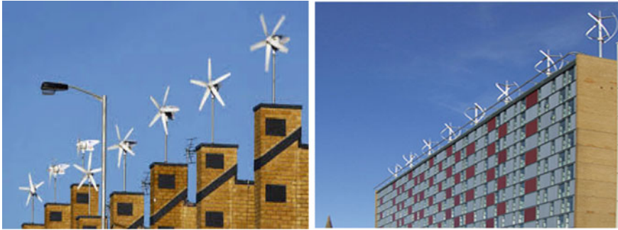
Fig. 9.10 Wind Turbine installed on Croydon City House, UK ( left ) and a community house in Kenya ( right )
