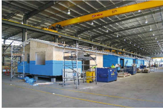
Fig. 3.8 Supporting Pads System on the factory floor. Each module is fixed on supporting pads and stays stationary until completion (Fleetwood AU)
