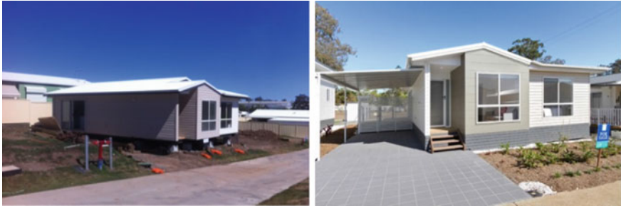
Fig. 3.17 Housing units installed on-site. Foundation types and connections are specified by engineers based on the soil conditions of the site installation
