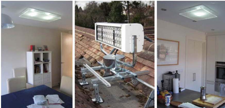
Fig. 9.25 Application of Parans daylighting system for a private residential home, UK
