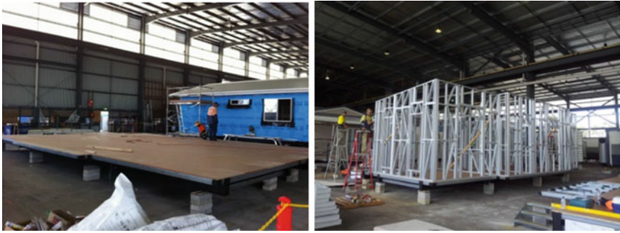
Fig. 3.12 Flooring and framing work for walls, ceiling and roof begin once the chassis is laid down. The cold formed light gauge steel frame and structure is designed to sustain cyclones up to 61 m/s
