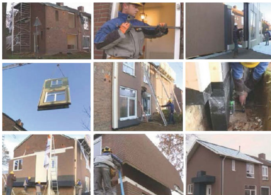
Fig. 10.18 Prefabricated elements designed for a fast renovation of social housing, Energiesprong or the Dutch experience (Energiesprong 2015a, b)
