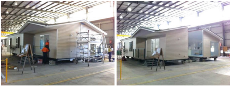
Fig. 3.15 Each manufactured home consists of two unit modules. After completion in the factory, modules are separated and prepared for transportation to site. Ply and strap bracing are applied to the side joints to prevent damage during lifting, transportation and installation on site
