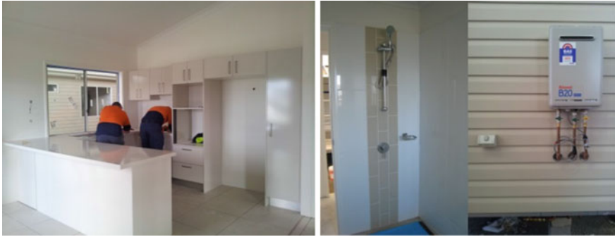
Fig. 3.14 Internal lining and finishes such as painting, tiling etc. are completed in the factory. All electrical fixtures, equipment, lightings, air conditioning system, plumbing fixtures and hot water supply unit are also installed in the factory. Module joints are the only remaining area to be completed on-site
