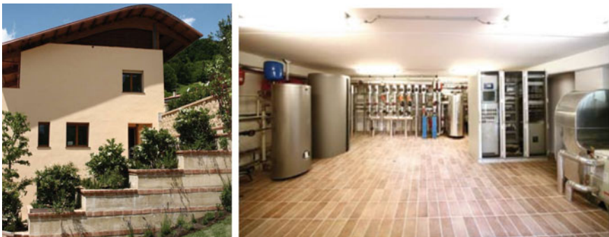
Fig. 9.14 (Left) Leaf House side view and (right) geothermal system fittings (Leaf 2015)
