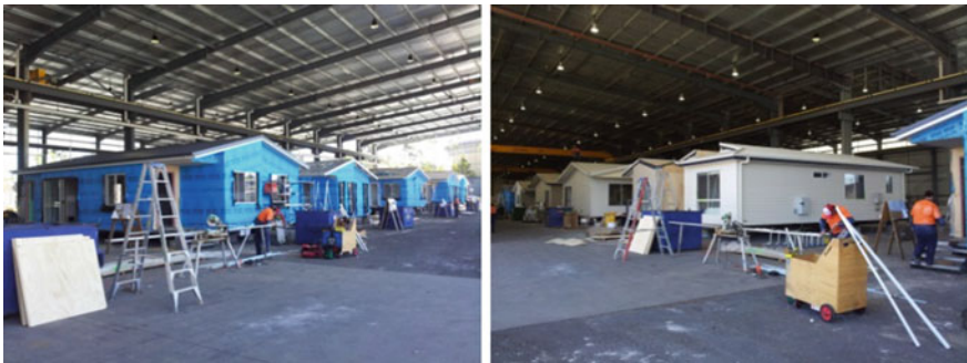
Fig. 3.13 External cladding and roofing are finished. Each building is tested by energy efficiency assessors to achieve a 6 star energy efficiency rating. The site location, building orientation, external and internal finish materials, colours, glazing, wall and roof insulation systems etc. are checked in the assessment processes
