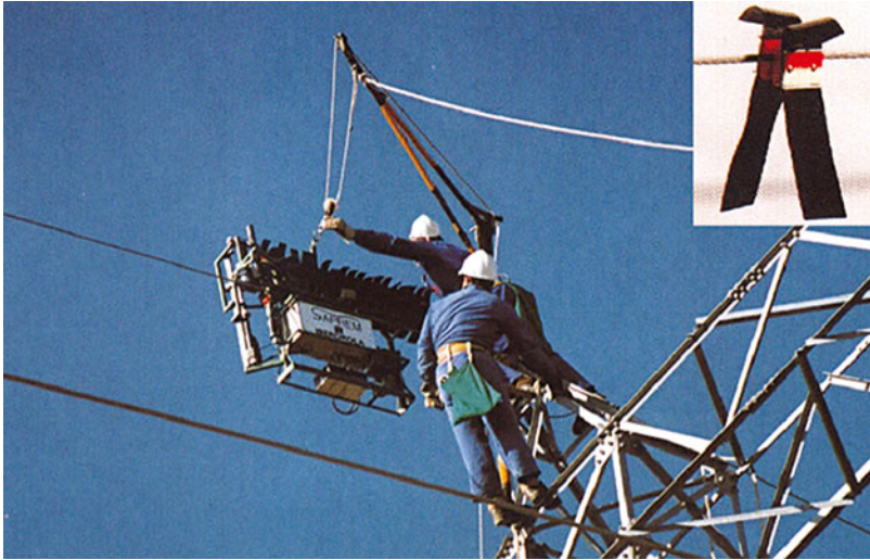
Figure 6.8 An example of a bird flight devices on the ground wire. A special trolley was developed to install the devices automatically on the wire (Spain).
