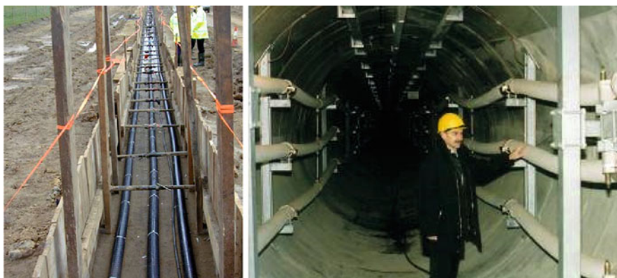
Figure 19.2 Left – one cable system direct buried in soil (from Cigré TB 338, page D.2); Right - two XLPE 400 kV cable systems in a ventilated tunnel, 2×1100 MVA, special application in cities (Berlin, picture APG).
