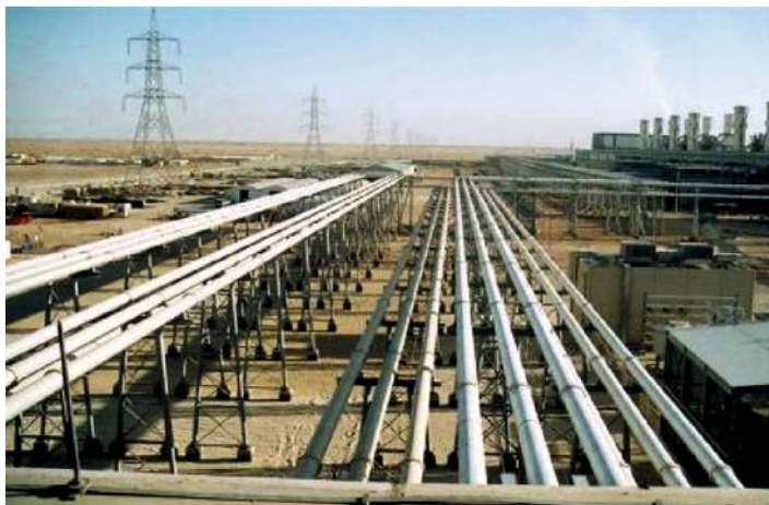
Figure 19.7 400kV GIL in Saudi Arabia, 780 MVA per system, installation above ground, connection of a power plant with the GIS (Cigré TB 218).
