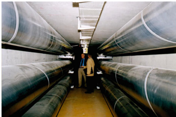
Figure 19.6 220kV GIL in Geneva/CH, energized in 2001, two electric systems in a tunnel, welded GIL of “2nd generation”, 2×760MVA (Picture APG).
