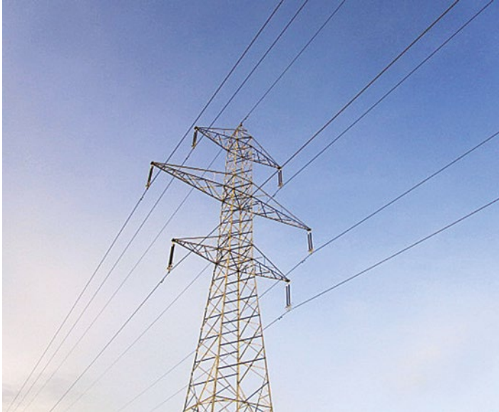
Figure 17.1 Typical 220 kV double circuit lattice steel tower.
