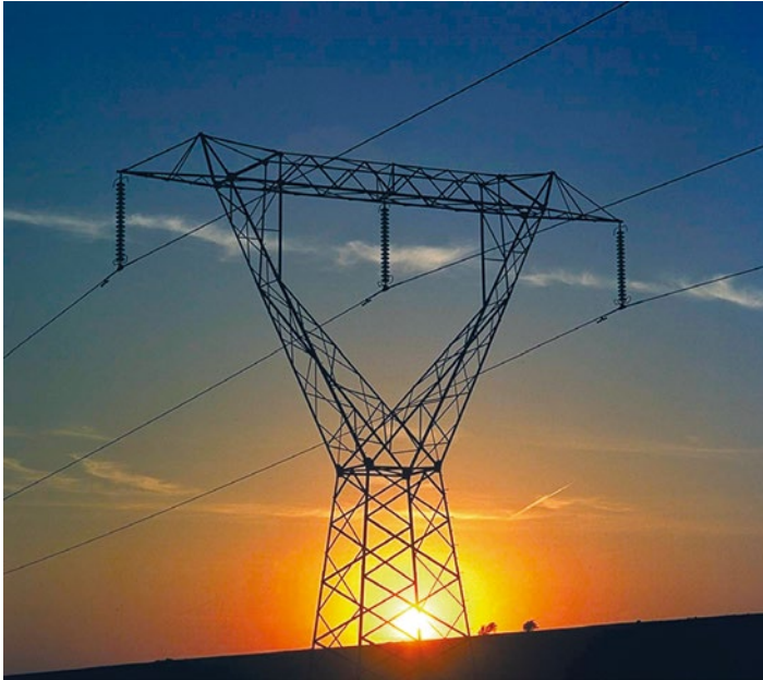
Figure 17.2 220 kV single circuit lattice steel tower.
