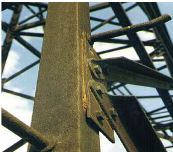
Figure 16.7 Corrosion at tower joints.
