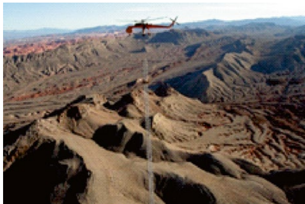
Figure 15.32 Helicopter Method – an entire guyed tower is air transported by the helicopter to its erection spot.
