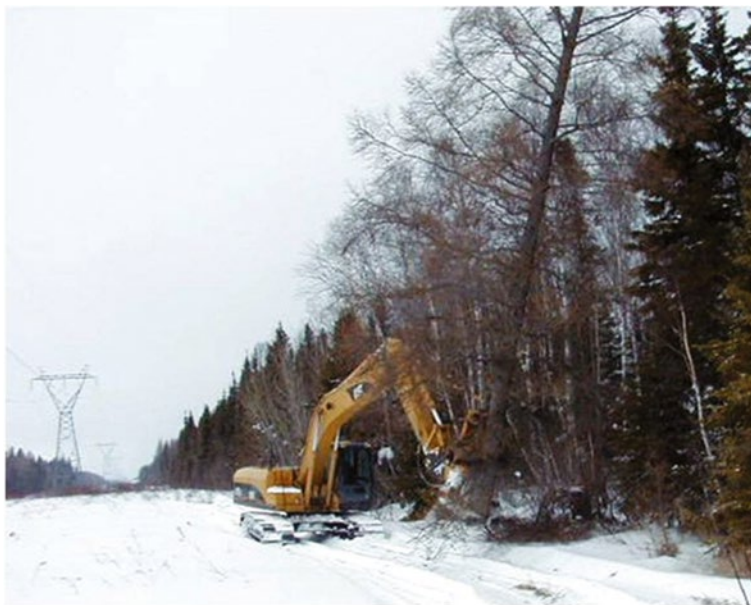
Figure 15.2 Feller buncher used to remove danger trees at the edge of right-of-way.
