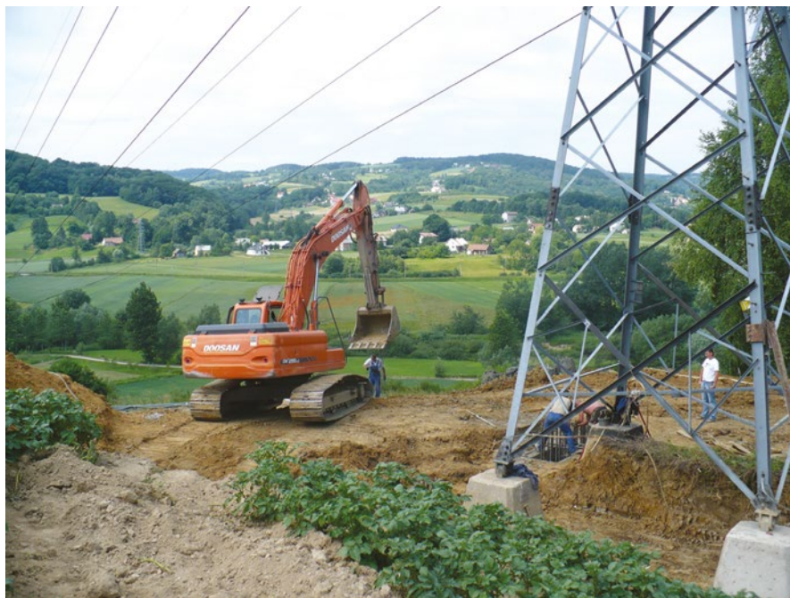
Figure 15.5 Hydraulic excavator during the work of strengthening the foundation of 110 kV OHL.
