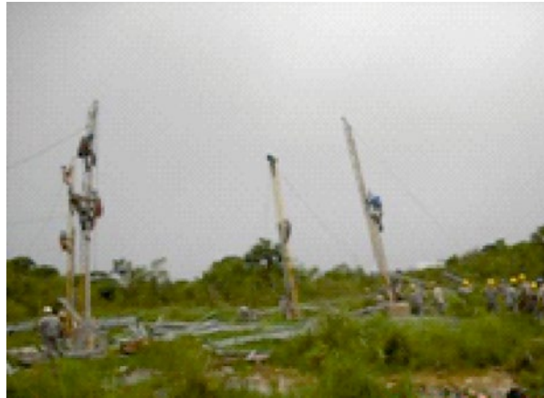
Figure 15.13 Build-up Method - Manual erection of a self-supporting tower aided by gin poles, in a swampy area; no access for cranes; no place for preassembling.
