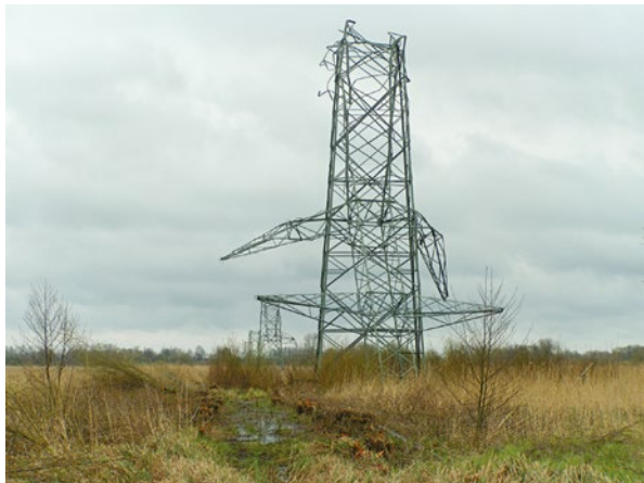
Figure 15.10 A view of the destroyed suspension towers of a 220 kV OHL.
