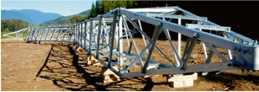
Figure 15.30 Helicopter Method – an entire guyed tower is preassembled on the ground and then lifted and air transported to its erection spot by the helicopter.
