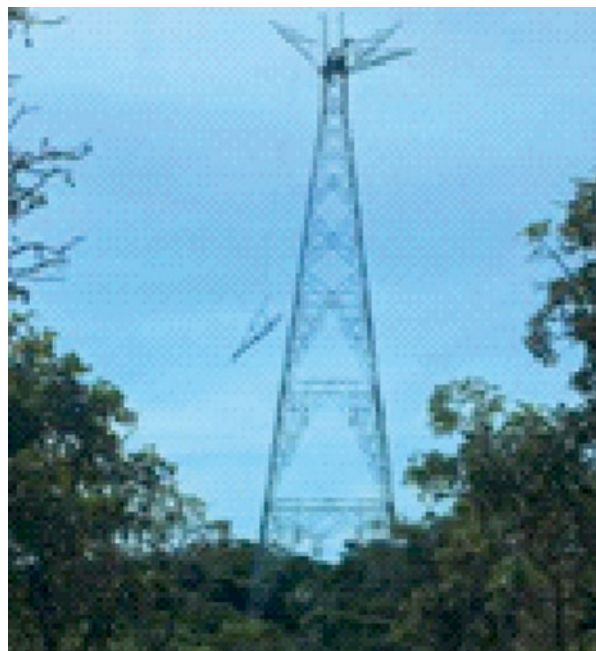
Figure 15.17 Section Method – a cross arm section of a self-supporting suspension tower is erected using a gin pole.
