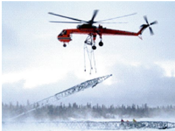
Figure 15.31 Helicopter Method – an entire guyed tower is rigged, tilted and then lifted and air transported.
