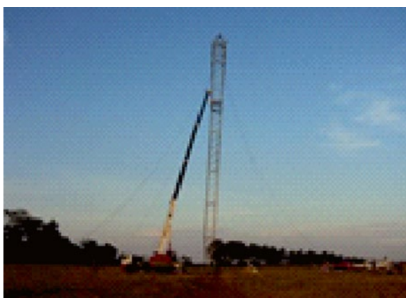
Figure 15.29 Tilt and Stand up Method – The tower is lifted and mounted in the central pin, the guy wires are anchored. (step 4).
