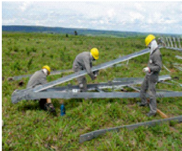
Figure 15.19 Section Method – a cross arm section of a tower is preassembled on the ground; this method speeds up the erection process.
