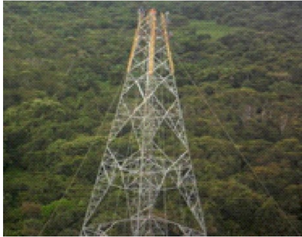
Figure 15.15 Build-up Method/Complementary -Manual erection of the upper part of a self-supporting tower aided by gin poles; tower height exceeded crane capacity range.
