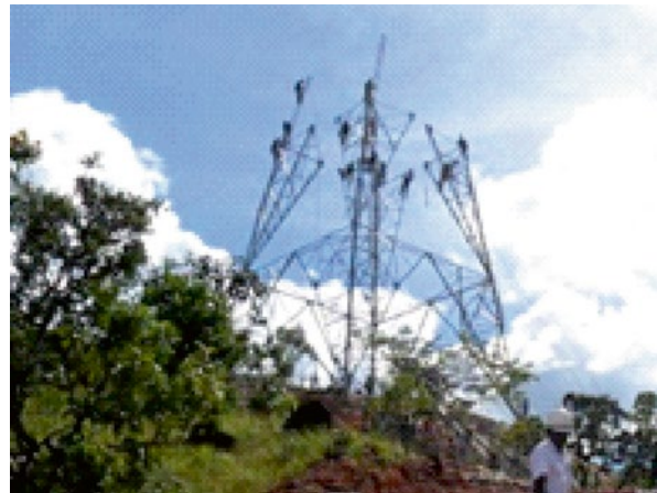
Figure 15.14 Build-up Method - Manual erection of a self-supporting tower aided by gin poles, in a mountainous area; no access for cranes; no place for preassembling.
