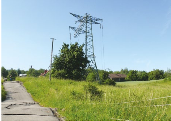
Figure 15.11 Tension tower destroyed and moved down about 14 m on a 110 kV OHL.
