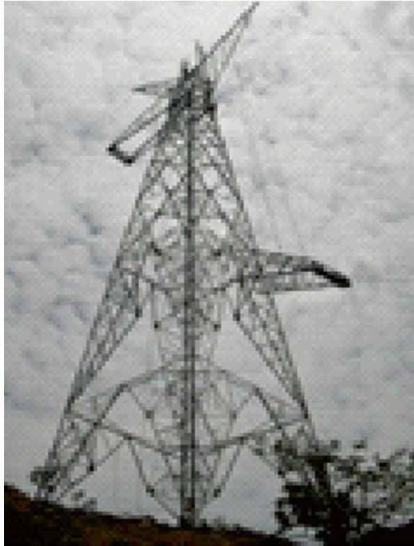
Figure 15.18 Section Method – a cross arm section of an angle tower is erected using a gin pole.
