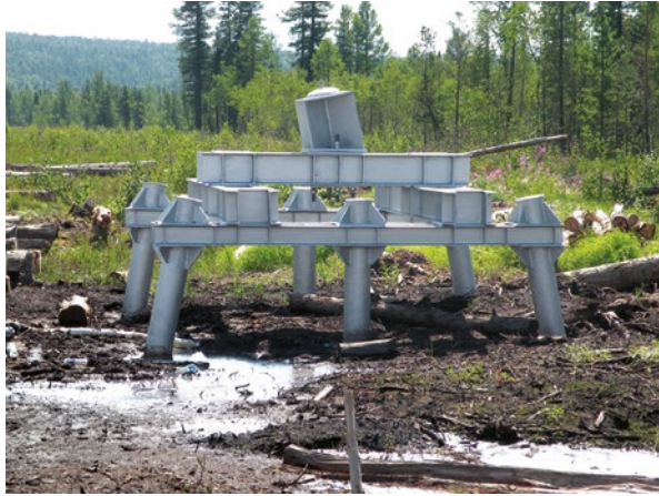
Figure 13.22 Steel screw piles with steel grillage – 500 kV portal guyed tower mast base.
