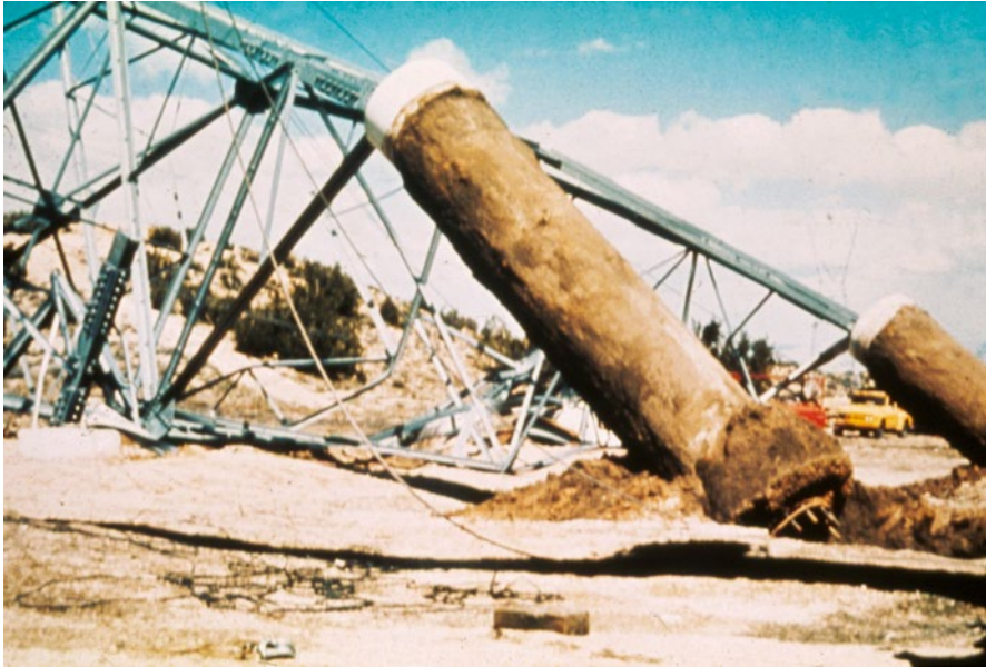
Figure 13.4 Failure of a 500 kV suspension tower drilled shaft foundation.
