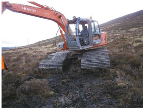
c) Use of low ground pressure excavator to reduce impact on peat soils
