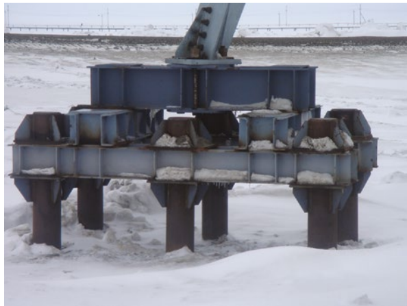
Figure 13.21 Driven steel tube piles with steel grillage – lattice steel tower leg connection.
