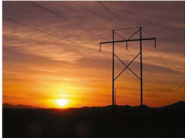
Figure 12.38 Pole structure for 110 kV line.
