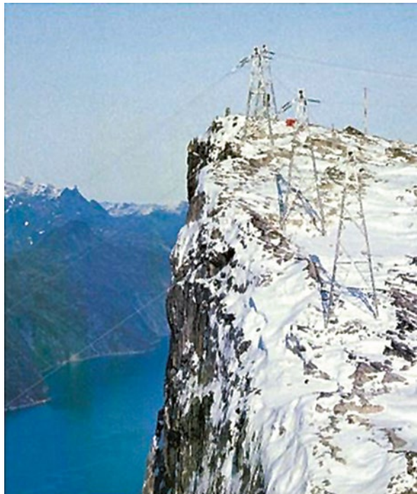
Figure 12.68 132 kV Ameralik Fjord Crossing, Greenland (5.37 km crossing span).
