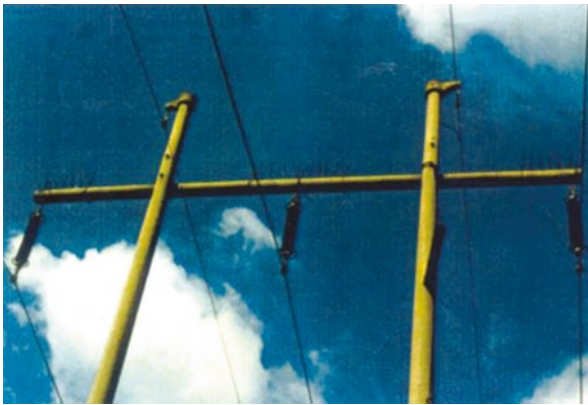
Figure 12.36 110 kV Concrete Pole.
